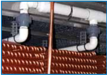
Evaporative Condenser Section
